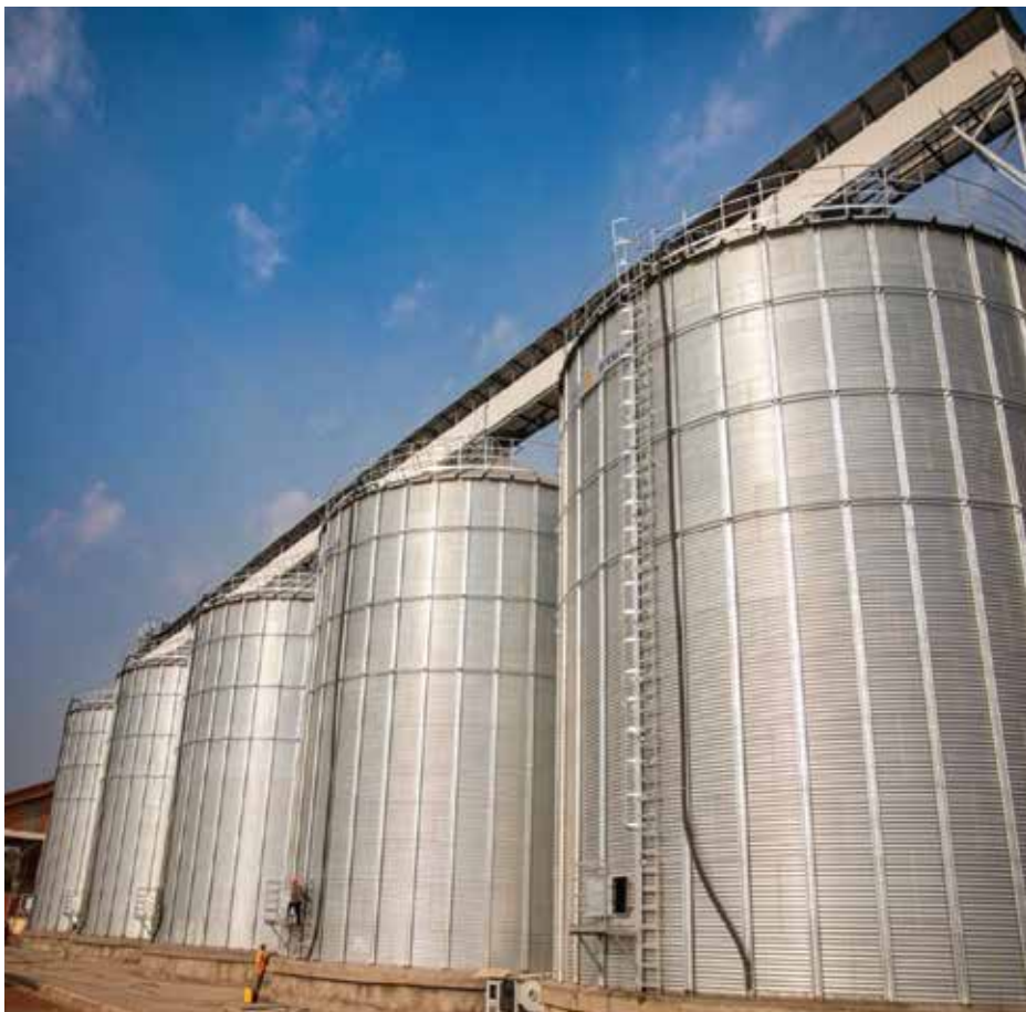
Five metallic silos installed in Nyagatare to increase the capacity of National Strategic Grain Reserve for maize grains from 8000MT to 18,000MT.
