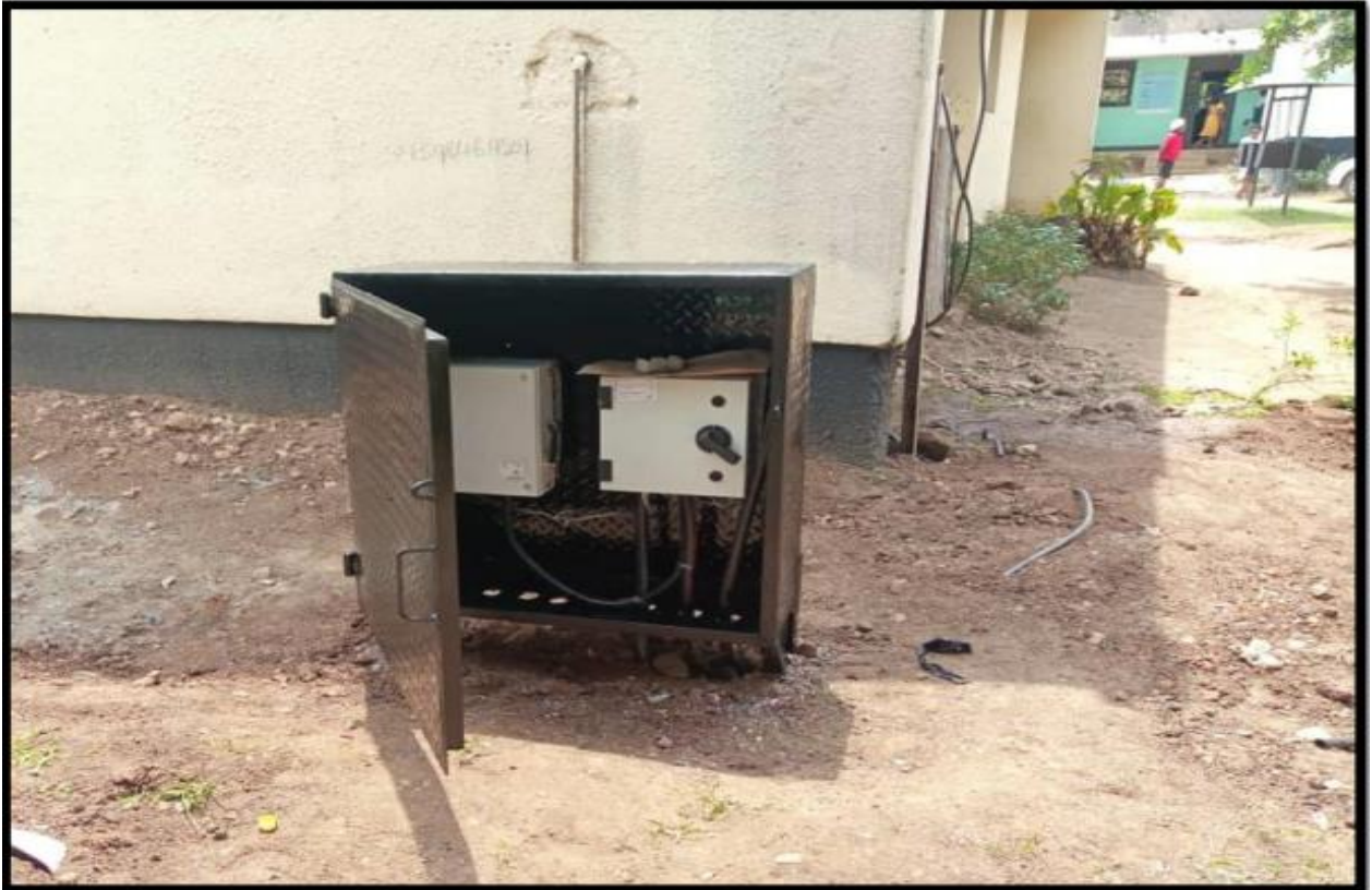
The control box with changeover and isolator Switches-Setup
